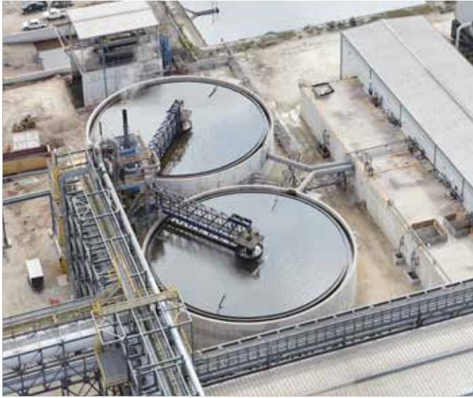
Fig. 1: Typical location of degassers for top gas scrubber weir and top gas scrubber cone return at the inlet to the clarifier(s)
