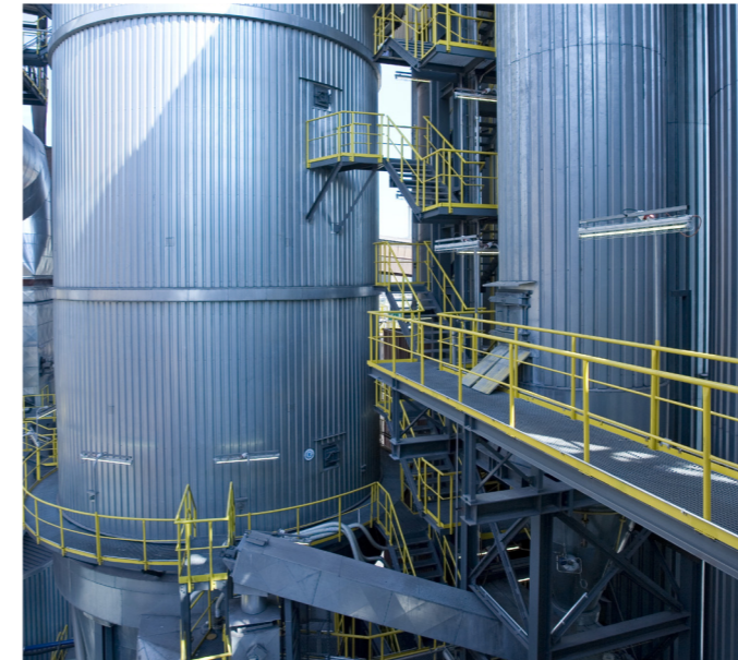
Gas conditioning tower
