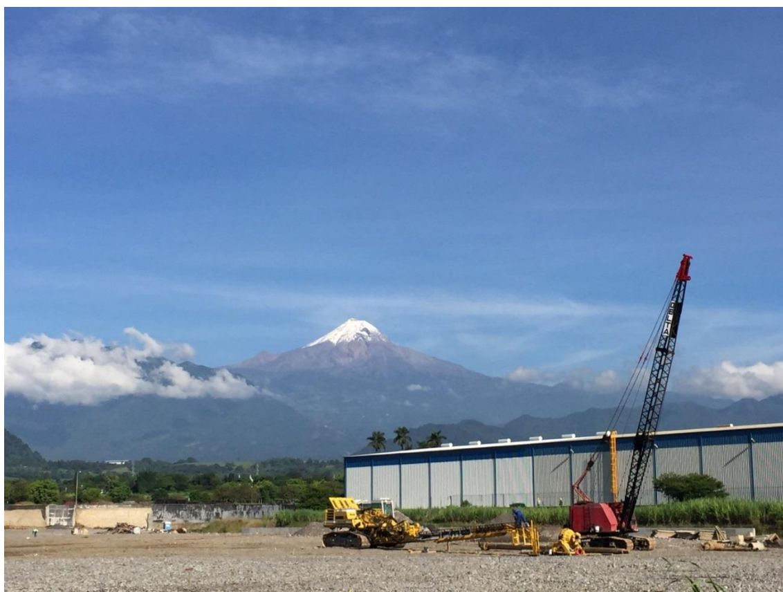
Excavation works for the first pier on Tyasa site for the combined galvanizing and color coating line
