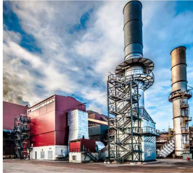
Bag-filter dedusting plant
