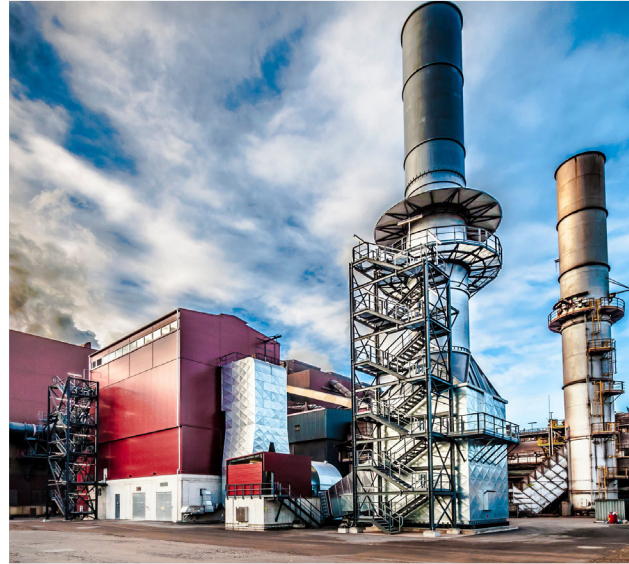
Bag-filter dedusting plant
