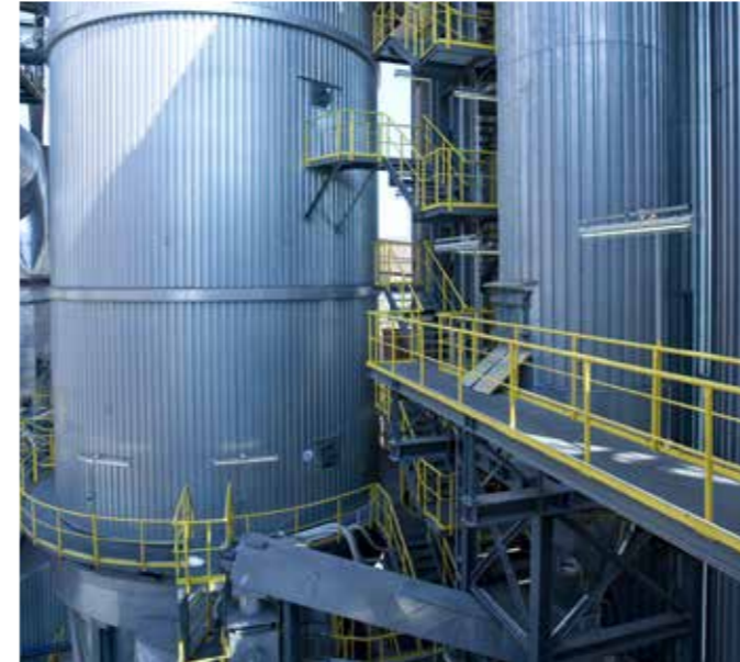
Gas conditioning tower
