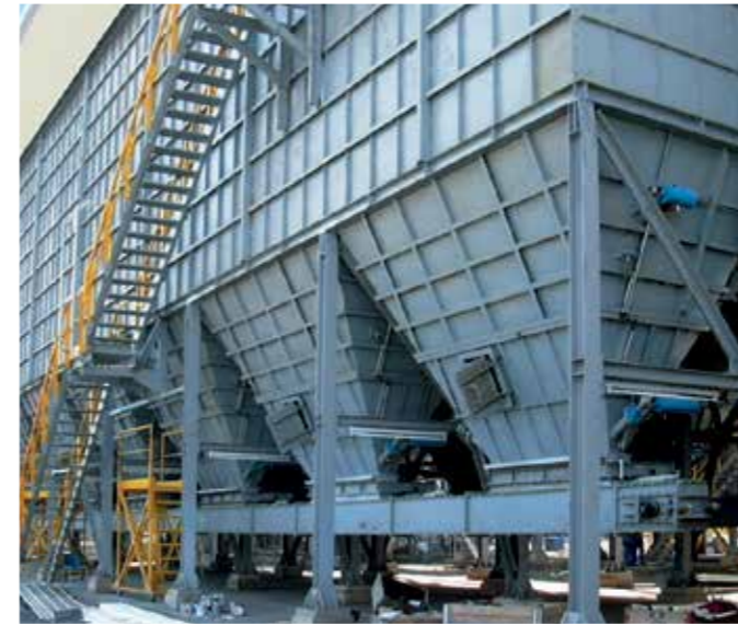
Hoppers with steep inclination avoid dust deposits
