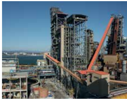
POSCO POHANG WORKS (KOREA) - FINEX® F-0.6M DEMONSTRATION PLANT
