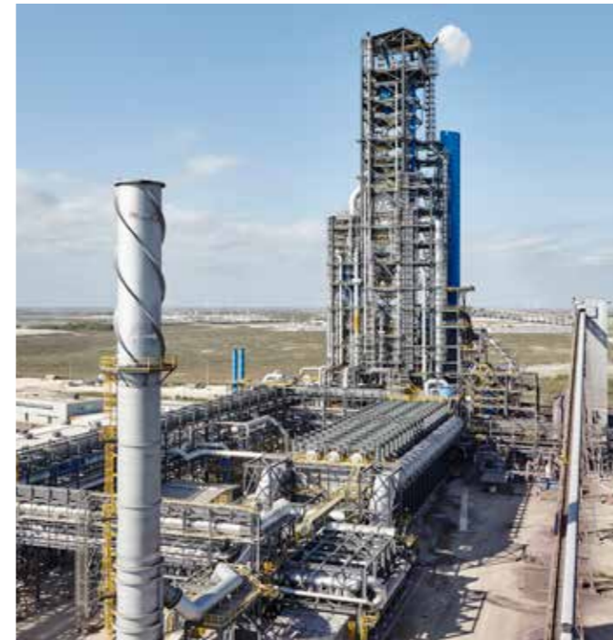
HBI plant tower and reformer
