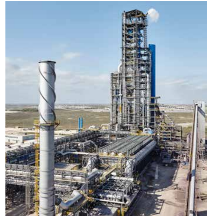
HBI plant tower and reformer
