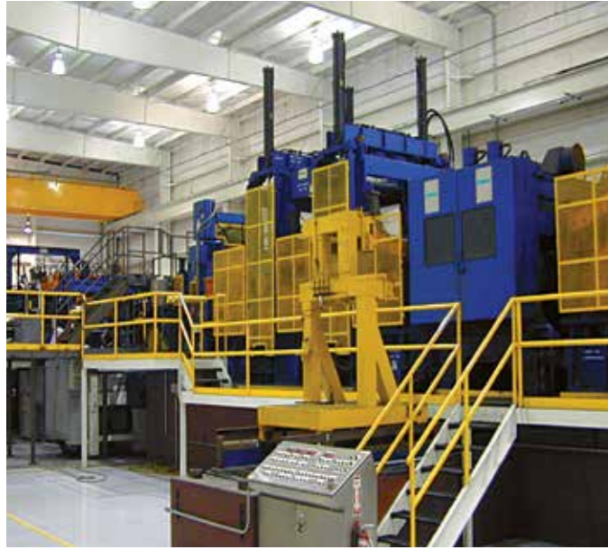
SB 50, Push pull pickling line
