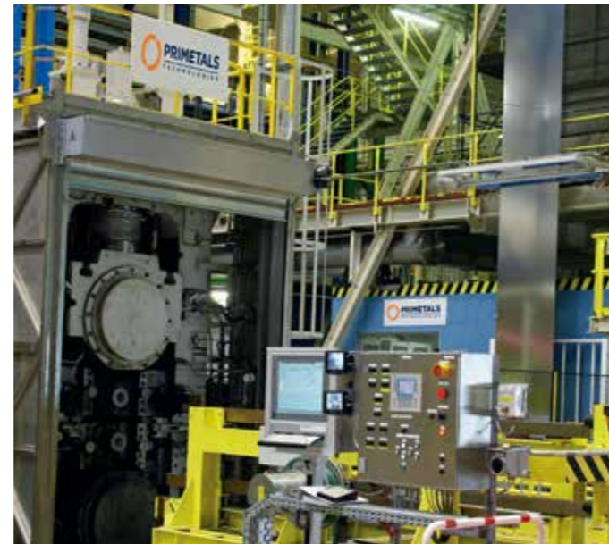
SPM 1200, Continuous galvanizing line
