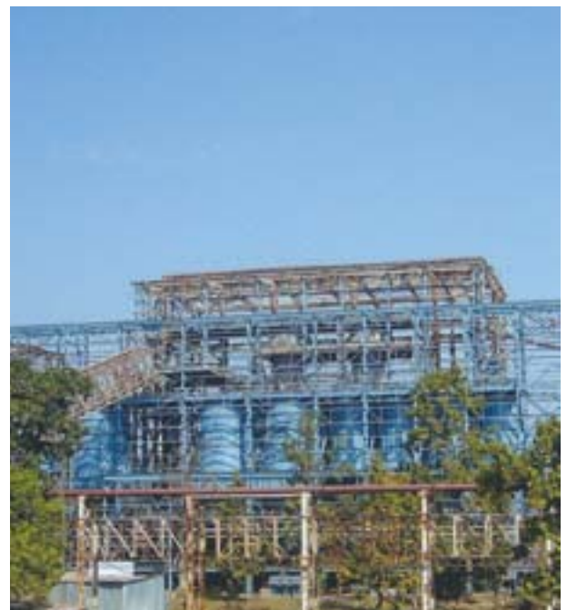
Construction of the world's first CPT plant at Pro Minerals Pvt. Ltd., Keonjhar, Orissa, India (February 2015)
