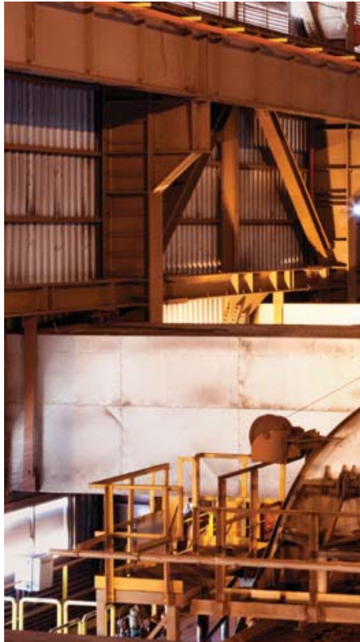
Selective Waste Gas Recirculation system installed at Dragon Steel Corporation, Taiwan
