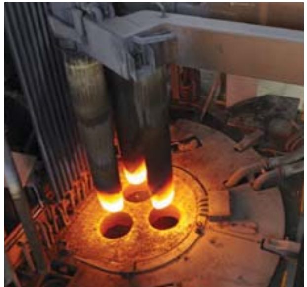
Current-conducting electrode arms installed in the 100-ton EAF Quantum Furnace at Tyasa, Mexico
