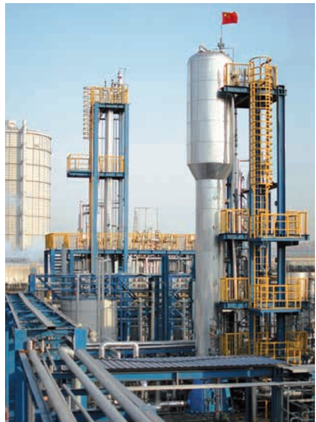
Example of a LanzaTech gas fermentation plant in China
