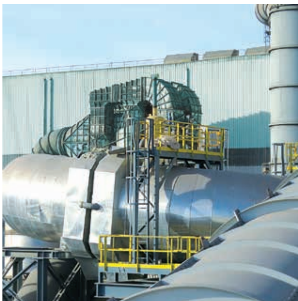
Industrial implementation of an EAF waste-heat recovery system for steam generation at Acciaieria Arvedi S.p.A., Cremona, Italy
