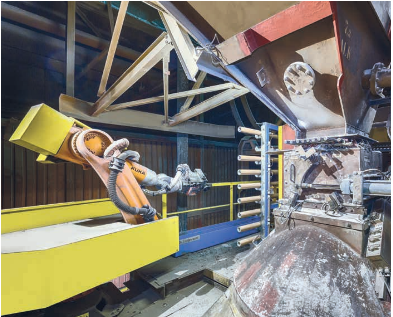
The robot system for fully automated handling of probes for the converter substance (voestalpine Stahl, Linz, Austria)
