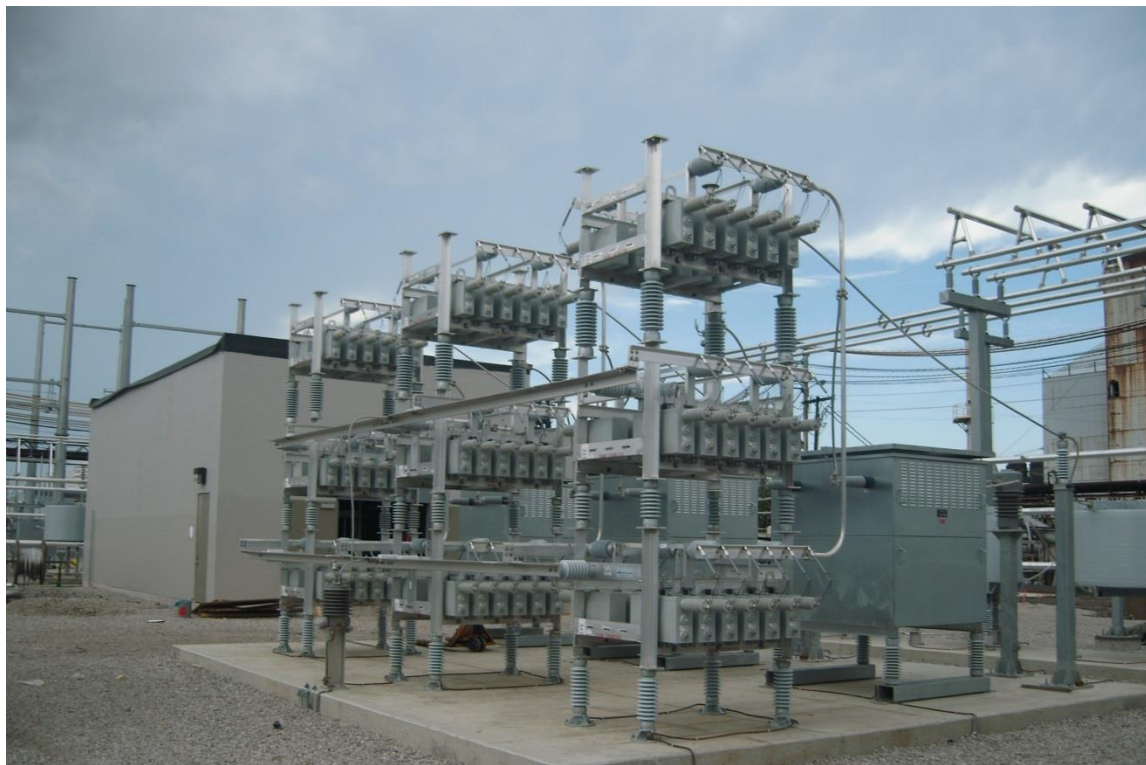
Substation with SVC system in building at left
