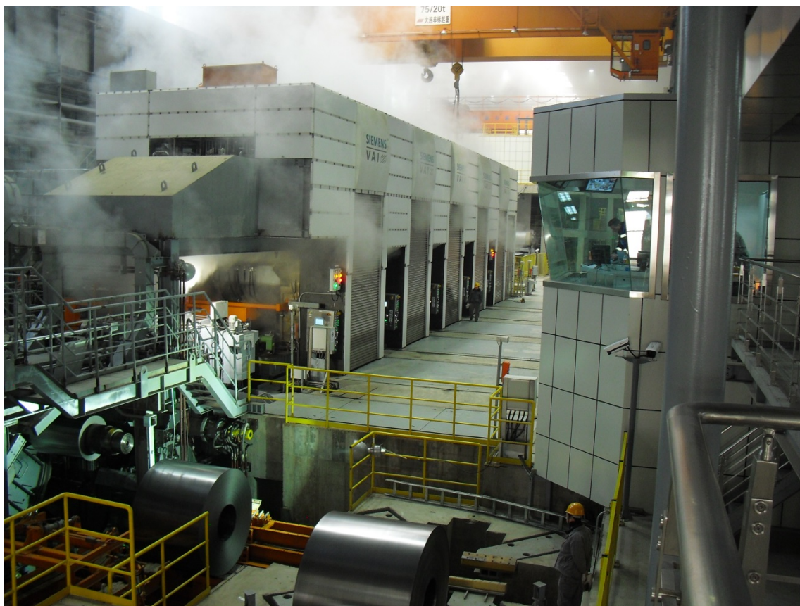
Cold rolling mill from Primetals Technologies at Tangshan Iron and Steel Group Co. Ltd.
