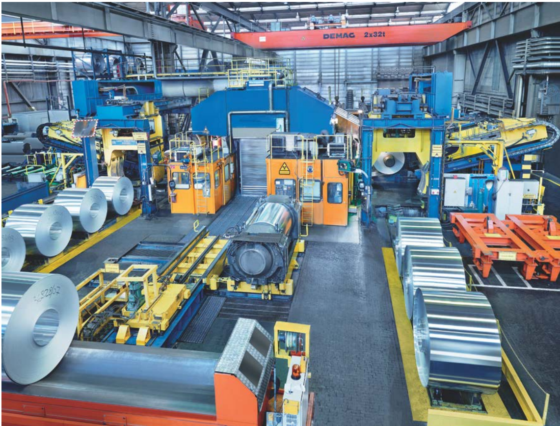
Strip production at AMAG rolling GmbH in Ranshofen, Austria. Primetals Technologies is going to modernize the entire drive technology of the four-high hot rolling stand (photo: AMAG rolling GmbH)
