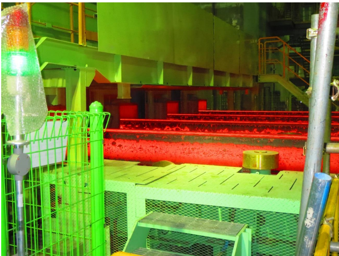
Continuous bloom caster from Primetals Technologies at Hyundai Steel in Dangjin, Korea
