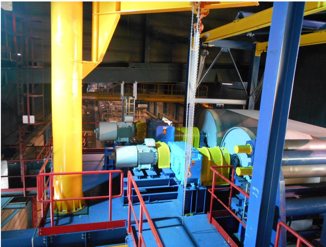
Modernized bridle area of the annealing and pickling line of Aperam in Genk in Belgium which was modernized by Primetals Technologies
