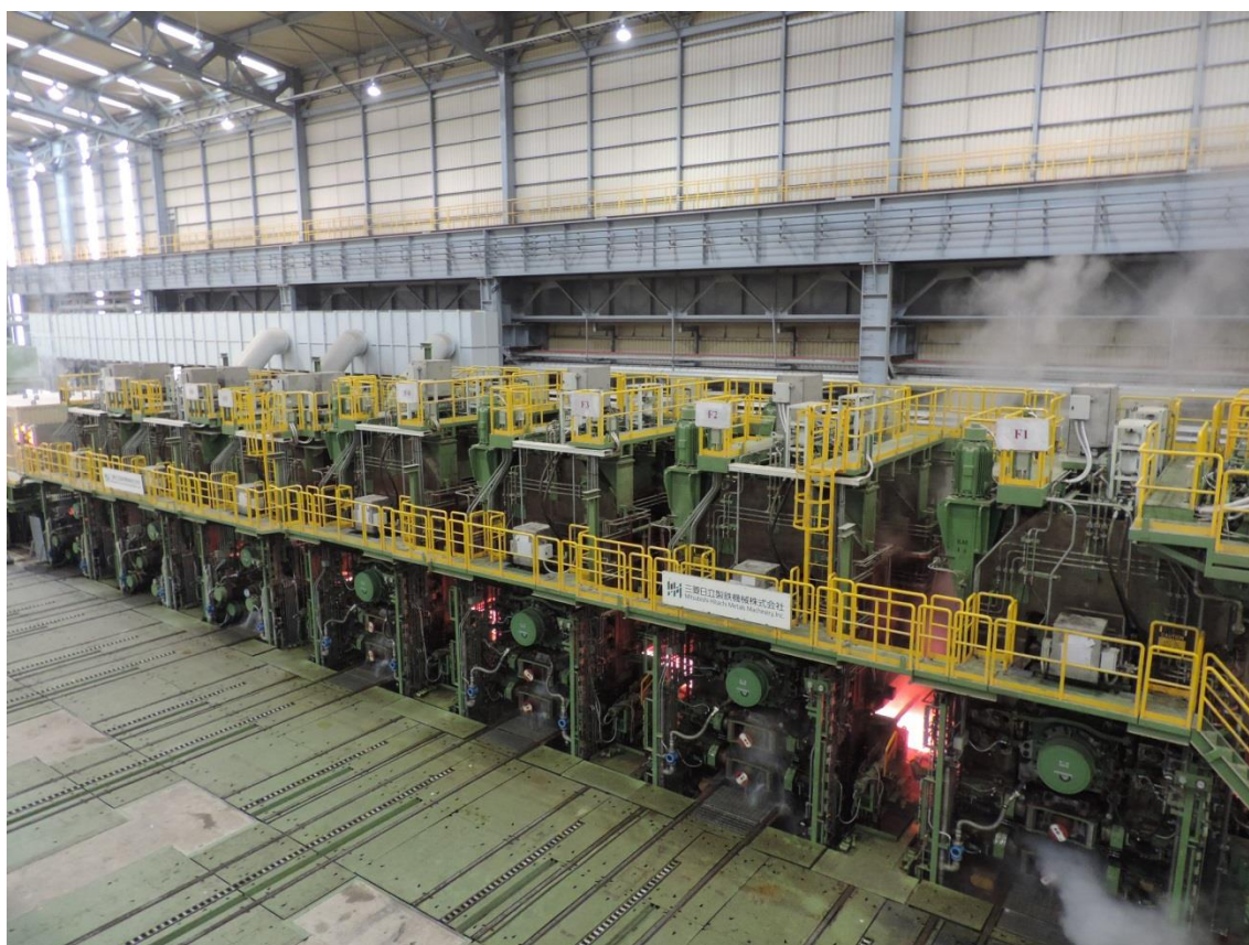
Finishing mill in the hot rolling mill from Primetals Technologies supplied to Formosa Ha Tinh Steel Co. in Vietnam. Four of the seven stands on the finishing mill are equipped with pair cross technology to optimize the progressive profile control. (Photo courtesy of FHS).
