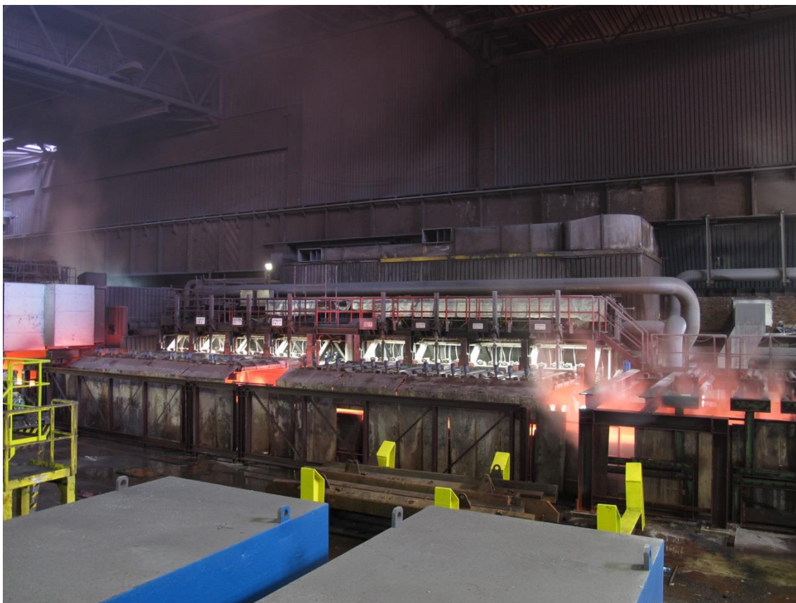
Power Cooling unit in operation
