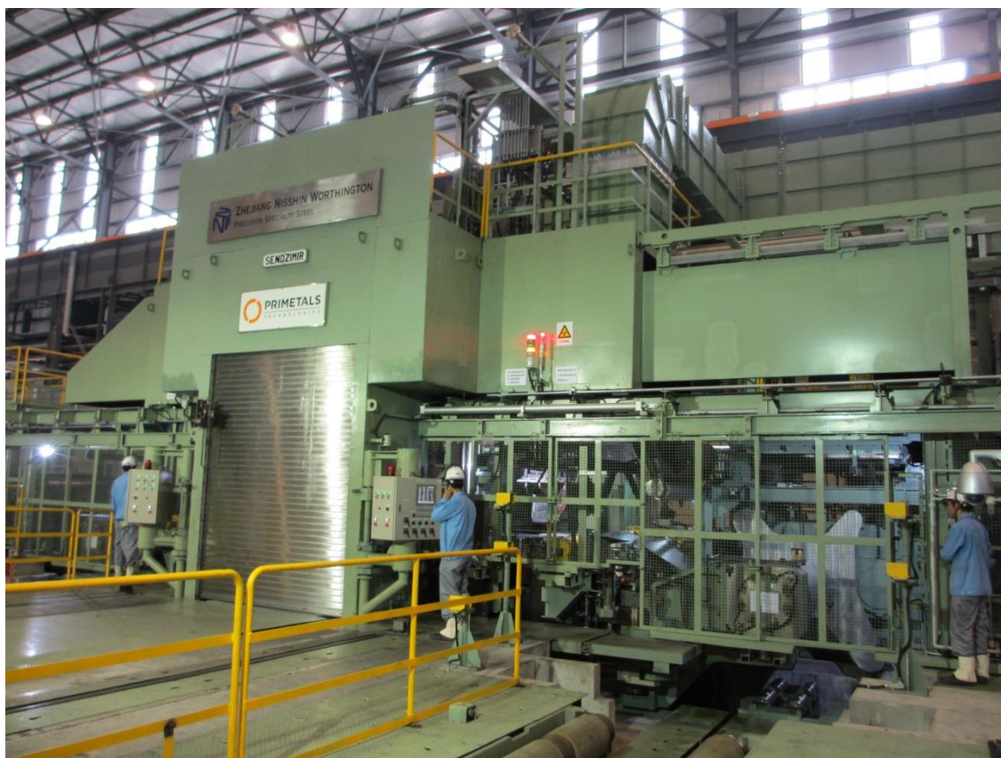
Front view of the Z-Hi reversing cold mill from Primetals Technologies at Zhejiang Nisshin Worthington Precision Specialty Steel Co., Ltd. in Pinghu, Zhejiang Province, China, which is exchangeable with a 4Hi mill for special steel.
