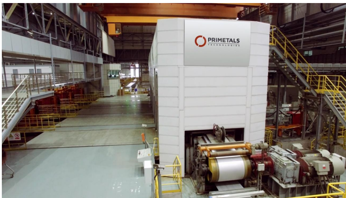
Cold rolling mill from Primetals Technologies at the Tangshan Iron and Steel Group Co. Ltd.
