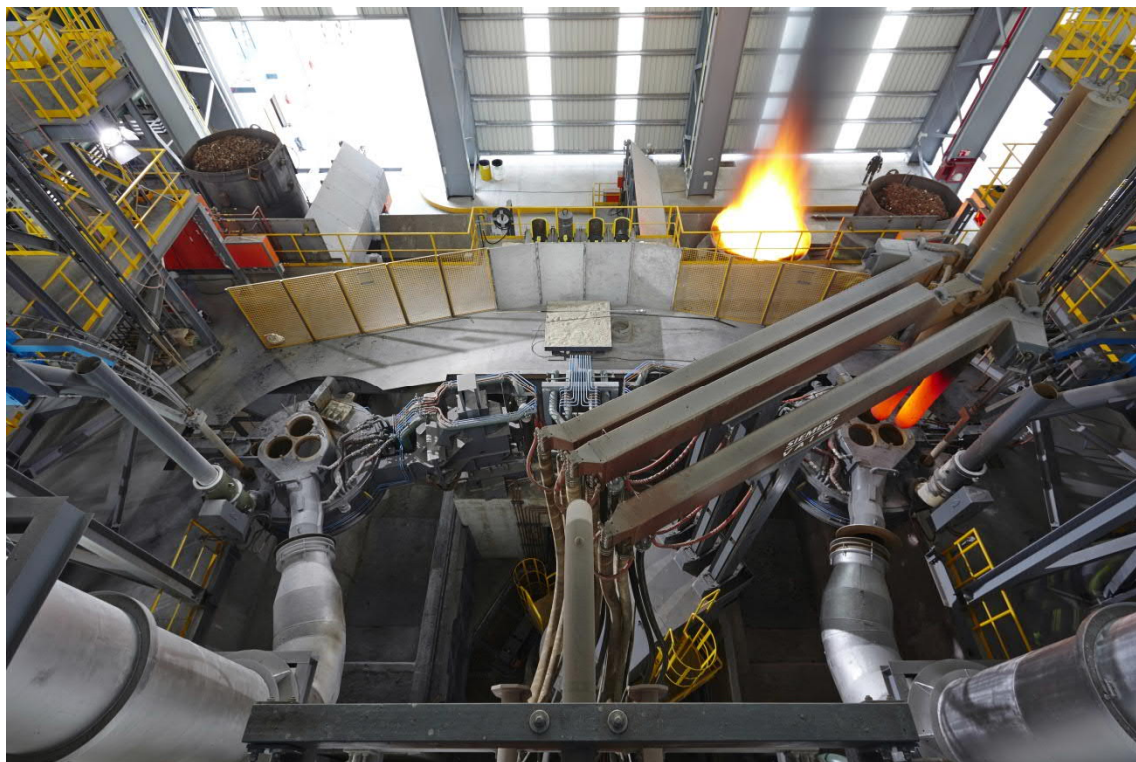
Twin ladle furnace from Primetals Technologies
