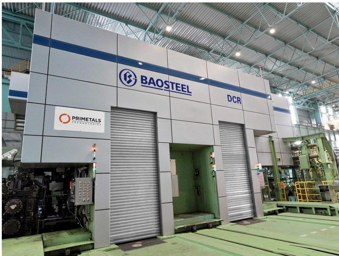
Front view of Baosteel's new DCR mill supplied by Primetals Technologies
