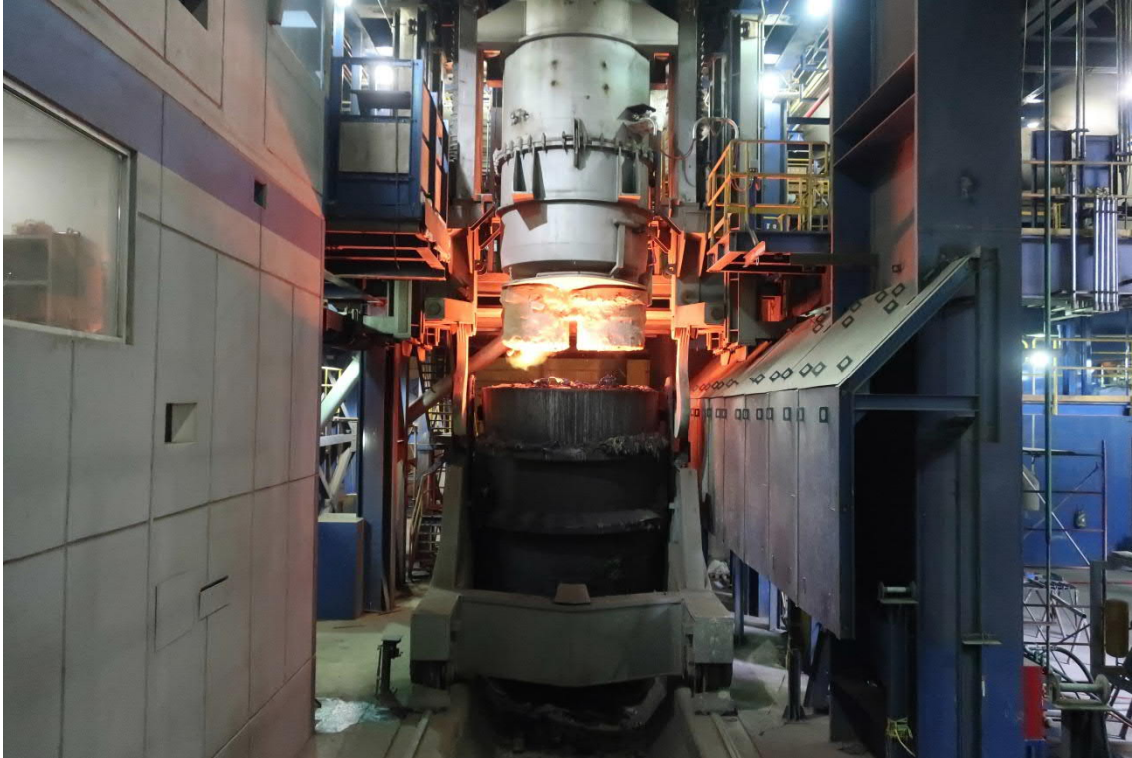
RH vacuum degassing plant from Primetals Technologies installed in the converter Steel Works # 2 of Altos Hornos de Mexico (AHMSA) in Monclova, Mexico
