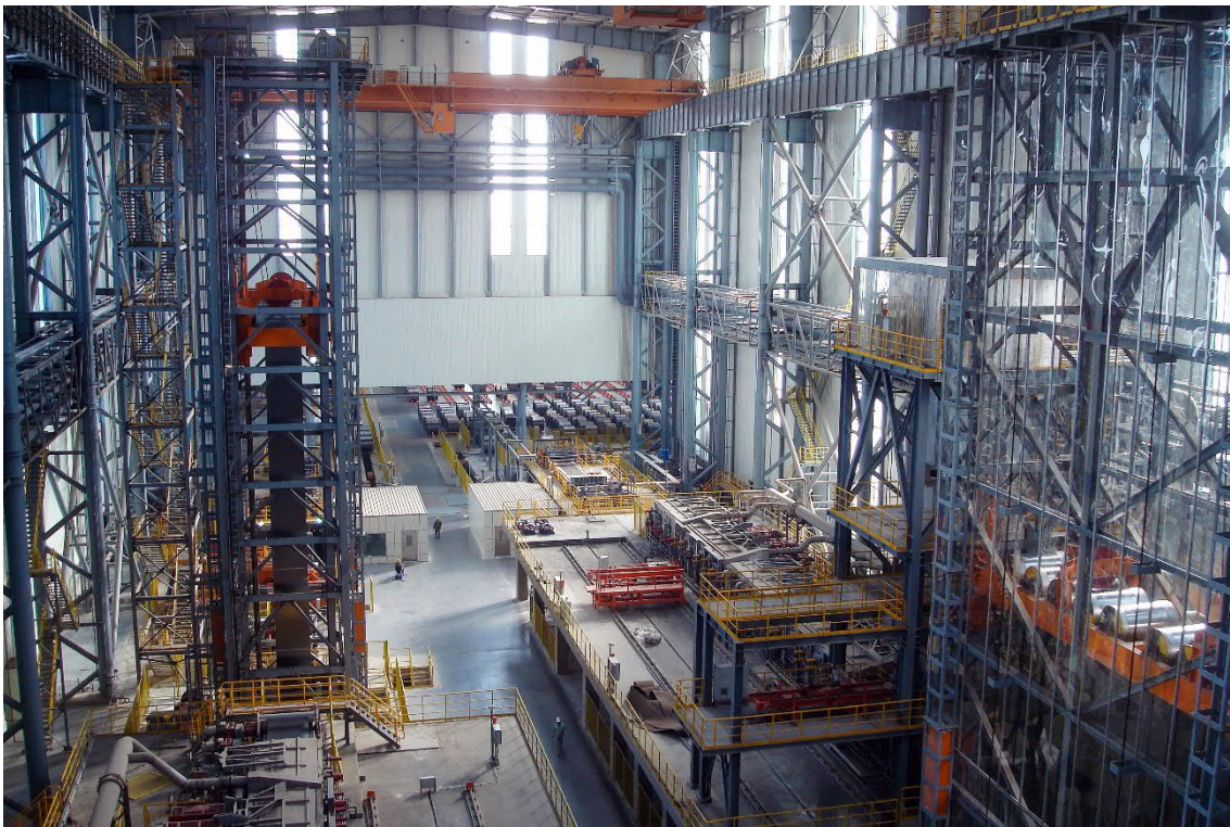
Continuous galvanizing lines CGL 5 and CGL 6 supplied by Primetals Technologies for the cold rolling mill of HBIS Tangsteel in Tangshan, Hebei Province
