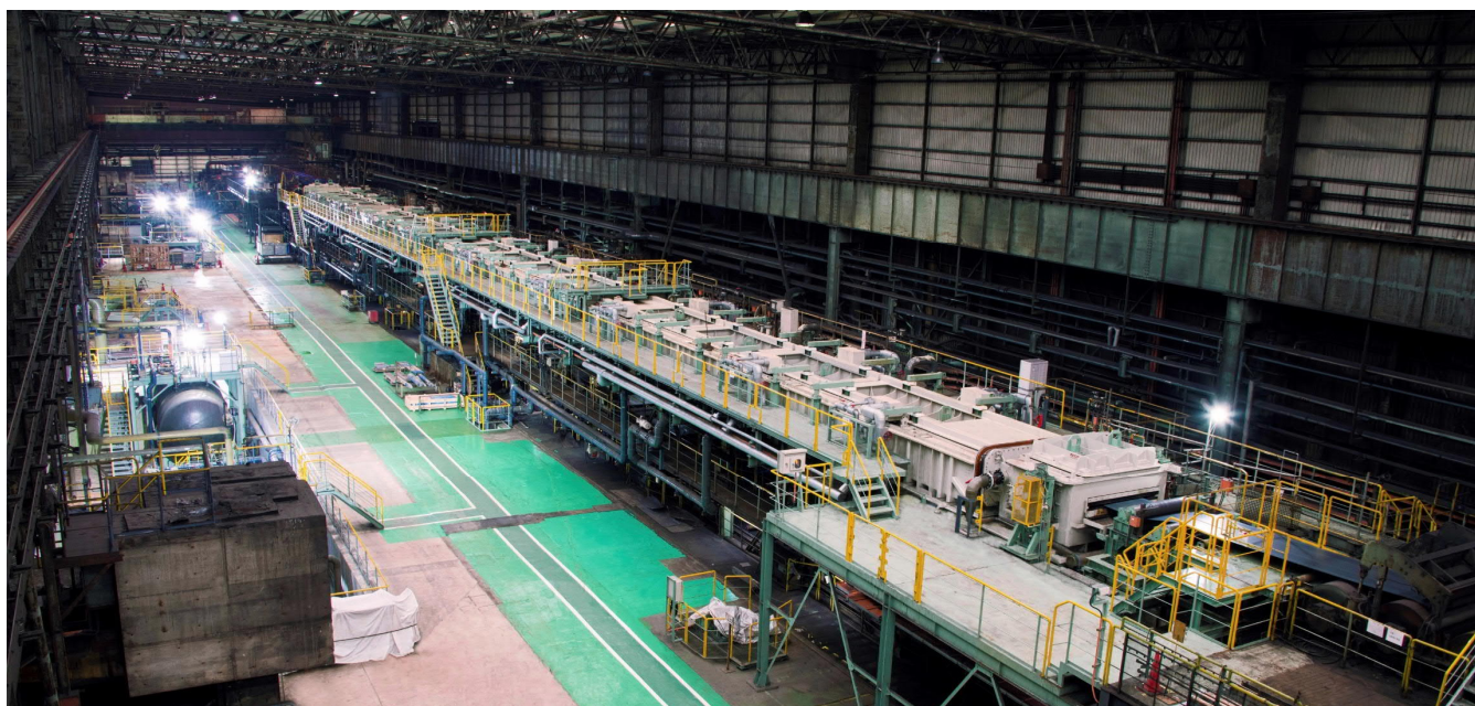
Pickling plant revamped with polypropylene iBox (July 13, 2020)
