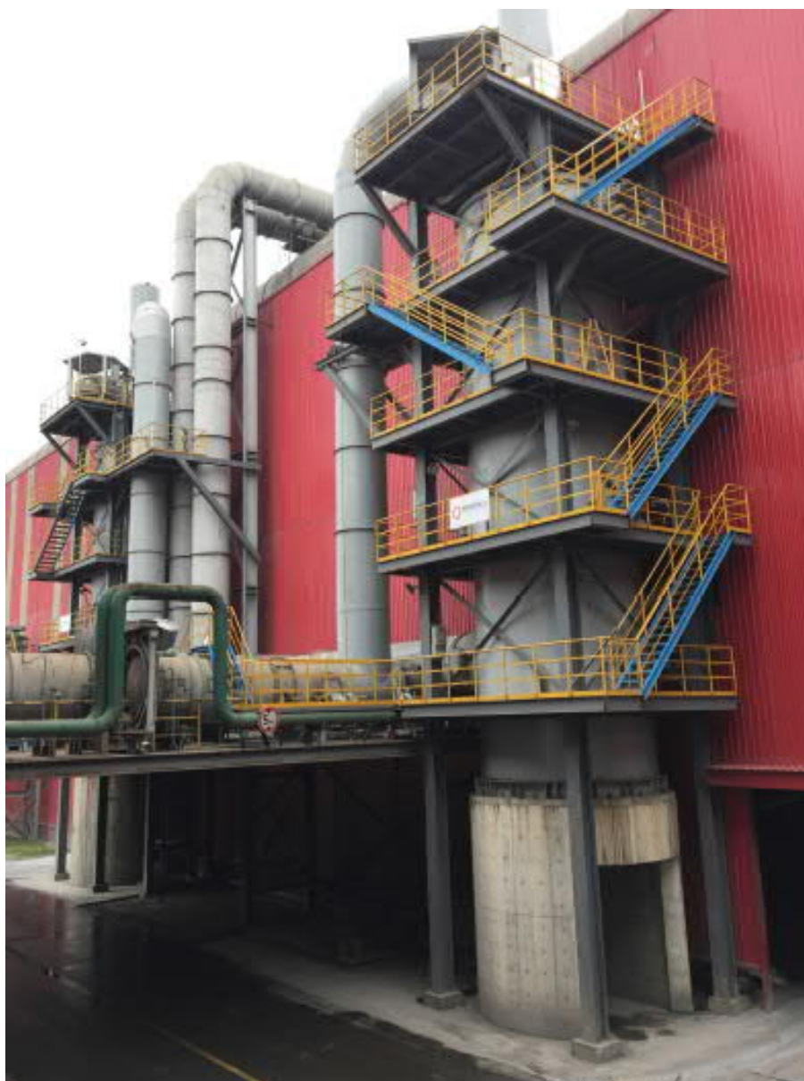
WESP towers from Primetals Technologies for BOF #1 and #2 at Changzhou Eastran Special Steel Co. Ltd.
