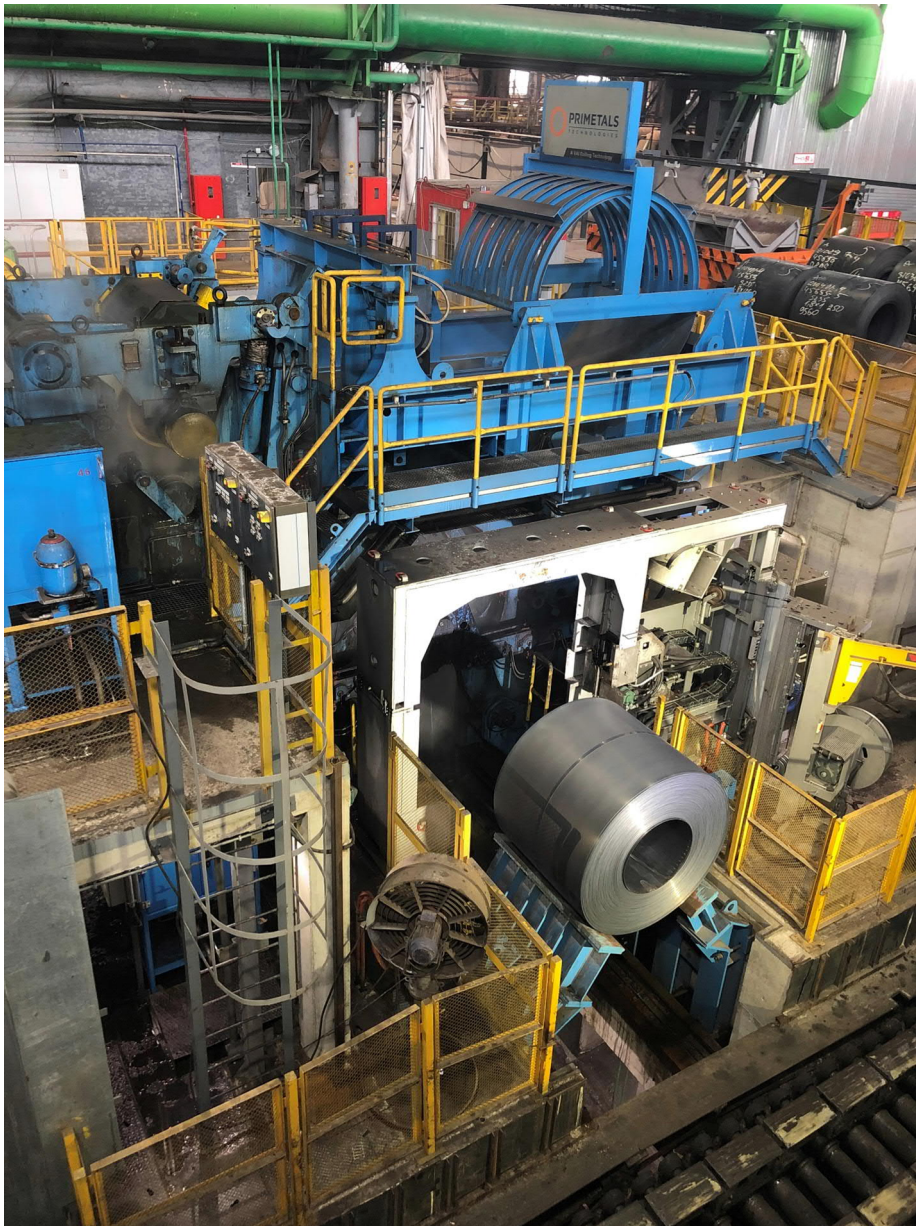
New downcoiler equipment at HSM 1700 at Ilyich Iron and Steel Works Mariupol installed by Primetals Technologies.
