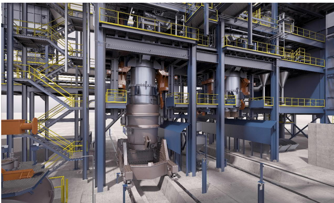
Twin RH degasser plant with CVL lifting system by Primetals Technologies
