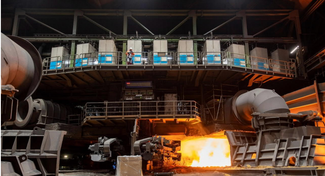
40 injection units located above the casting platform Duisburg blast furnace 'Schwelgern 1' © thyssenkrupp
