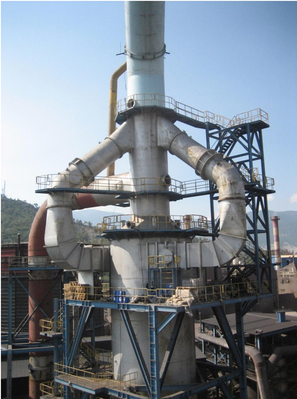
An operational 6.5m Tri-Ax Cyclone installed on a European Blast Furnace
