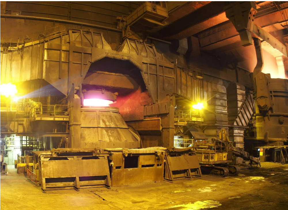
Charging of the new LD converter at ArcelorMittal's steel plant in Gent during first heat.
