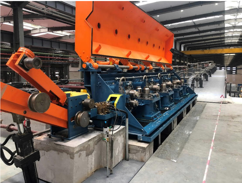
Copper rod mill from Primetals Technologies.
