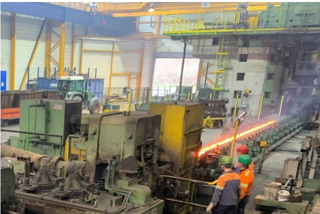
Primetals Technologies has modernized the automation system at BGH Edelstahlwerke's roughing mill.
