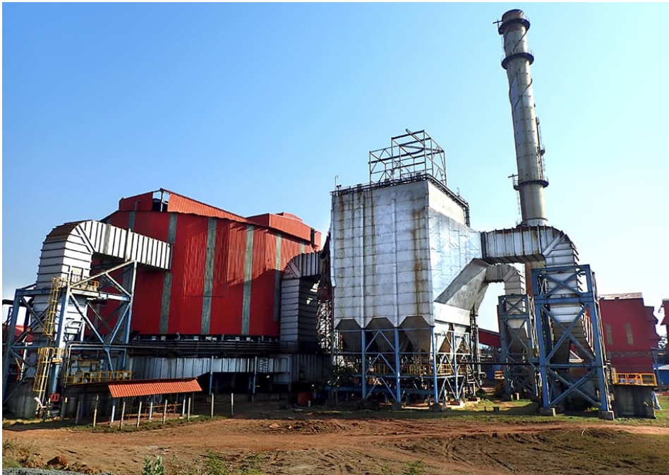
The circular pelletizing plant from Primetals Technologies at EMIL's premises in India.
