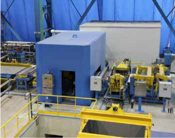
Welder Recoiling and Inspection Line, USS Kosice, Slovakia
